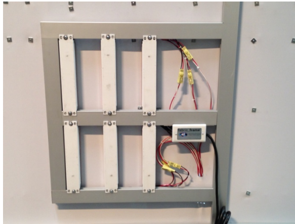
Power Supply Rack (Step 7)
